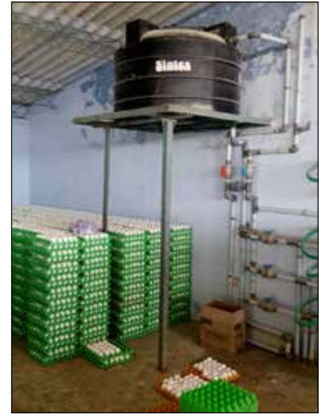
Figure 12. Having the water tank inside the house keeps the water cooler.
